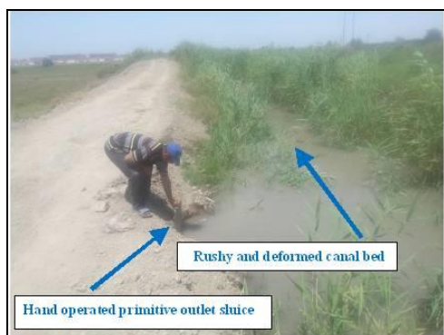
Figure 6. Turnout from the secondary canal, Salyan (2013).
